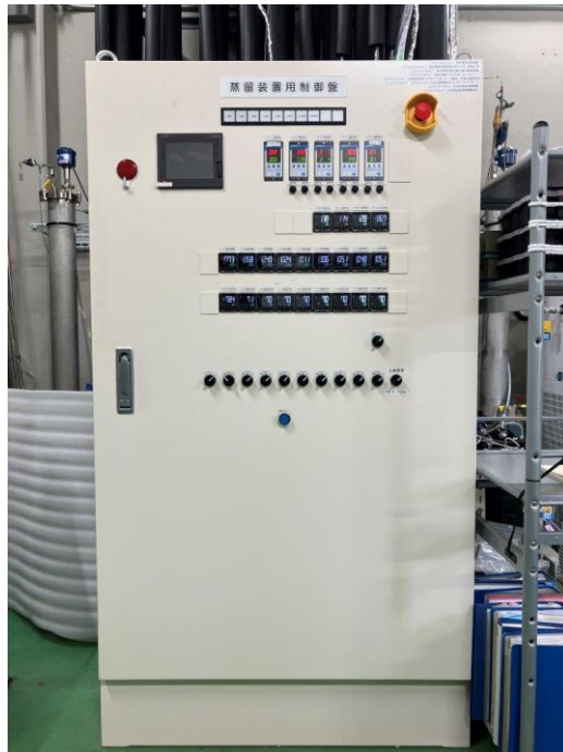
Heavy water reconcentration equipment (exterior view)
