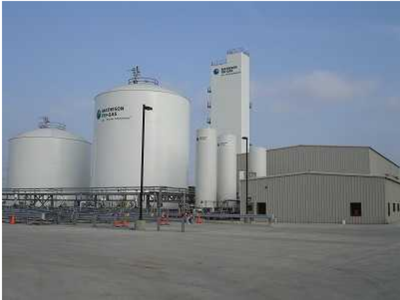
View of the plant at Vernon, California
