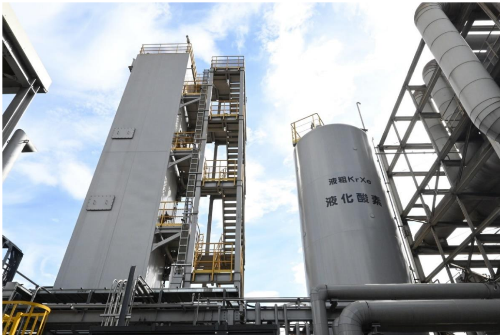
Newly-installed rare gas production facility
