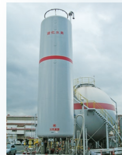
液化水素貯槽 設計圧力:0.97MPaG 貯液量:42.3m 3 Liquid hydrogen storage facility Design Pressure: 0.97MPaG Liquid Storage Capacity: 42.3m 3
